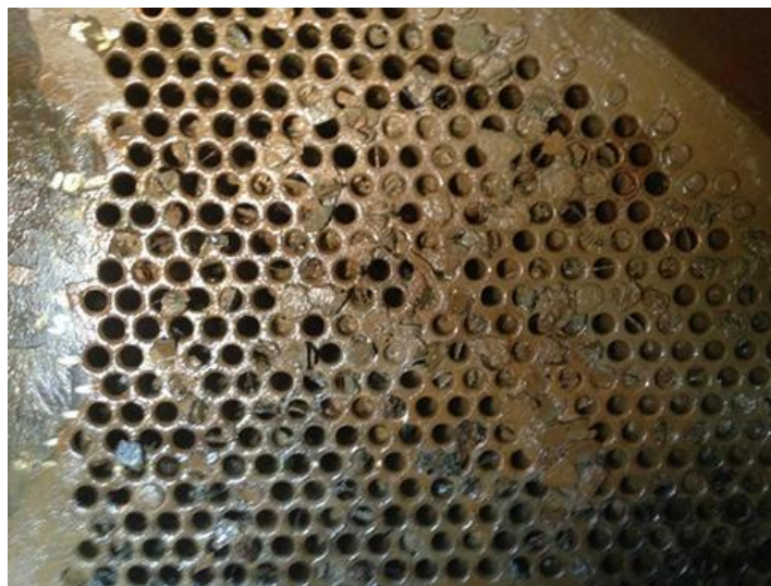
Figure 6-The Fouling on condenser tubes
